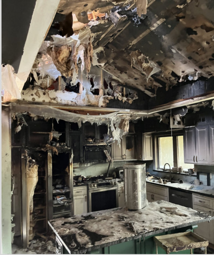
February 6, 2024 - Structure Fire 853 North 73rd Street Incident #24-001117
